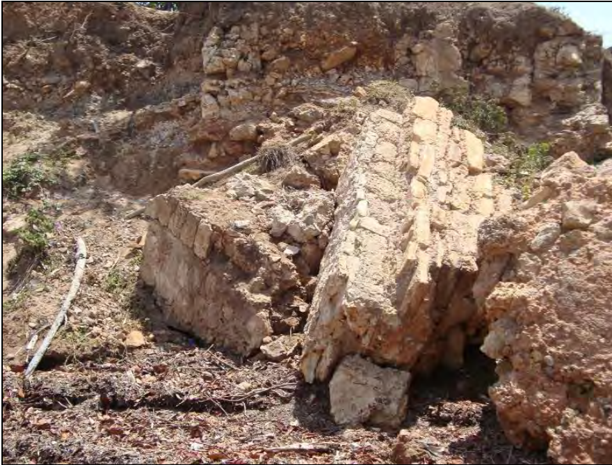
Figure 2: Damage from the Seawave action
